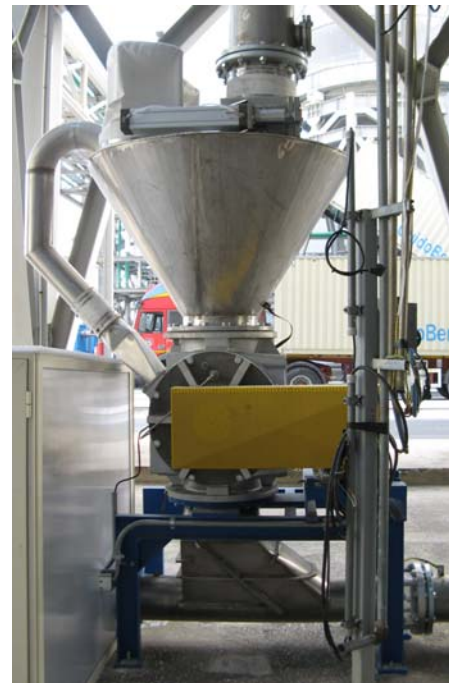
Rotoveyor for PET chips - Flow rate 45 t/hr - 160 m
