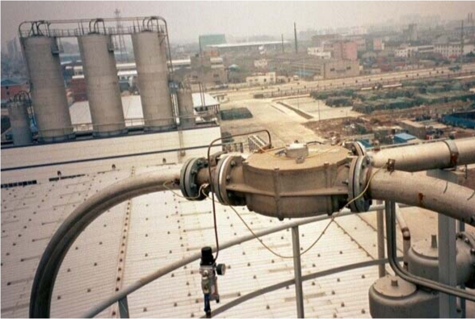
◀ MAB diverter valve size 150 installed in a pipeline conveying PTA powder with Nitrogen.
